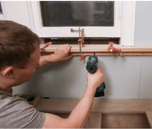
Window locates the top nailer. Clamp the backrest cap in place to set the height of the angled top nailer, then screw the nailer to the wall at each stud location.
