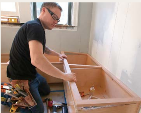
Flush it up. Set the top frames in glue, and align all outside edges flush to the face of the carcasses before fastening with finish nails.
