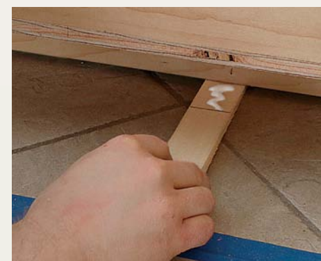
Help shims stay put. Stack shims to fit, then remove and coat with glue. Reinsert the stacks, let the glue dry, and trim the stacks flush.
